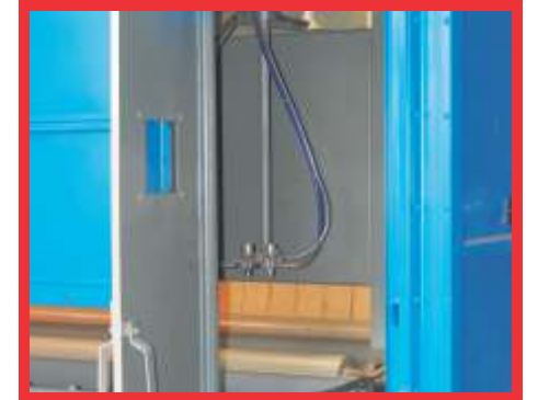
PAINT SPRAY BOOTH
